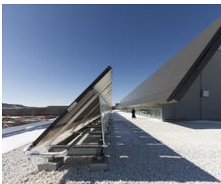
Solar Wall and Solar Thermal Collectors - Photo Credit: Peter A. Sellar
