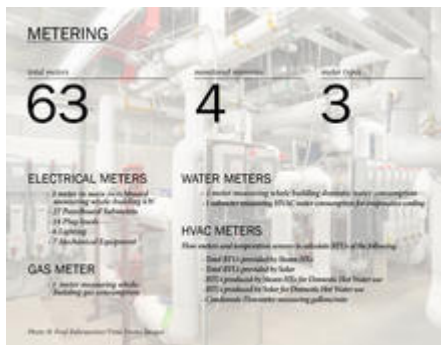
Metering - Photo Credit: Photo - Fred Fuhrmeister/Time Frame Images
