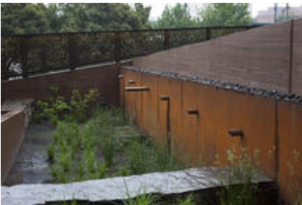
Another view of custom rainwater collection and stormwater treatment system. - Photo Credit: Sally Schoolmaster
